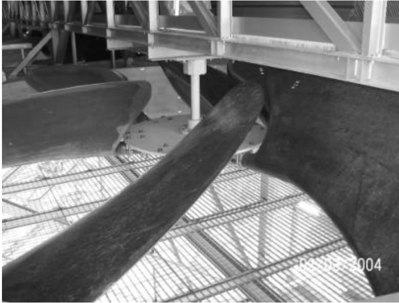
Figure 6: view of one ACC fan manufactured by the english Howden declaring its SX cooling fan as “the world's quietest, by far” (to not nullify its acoustical performance all the ACC electric motors drivers and gear-boxes have been decided to be acoustically enclosed)
